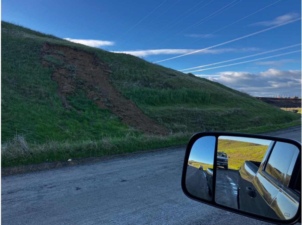
Figure 5: Phase I Northwest Slope erosion (Feb. 2025)
