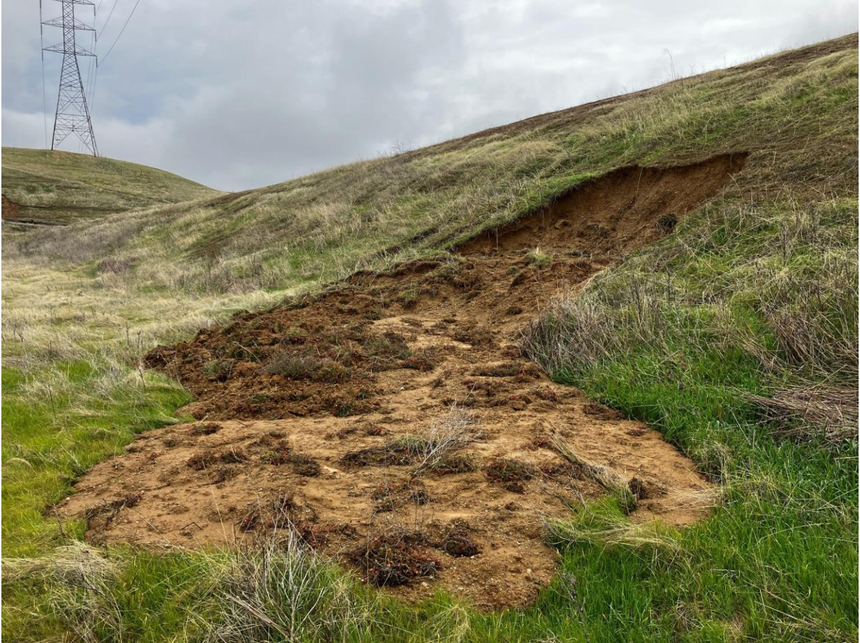
Figure 1: Phase I West Slope erosion (Dec. 2024)
